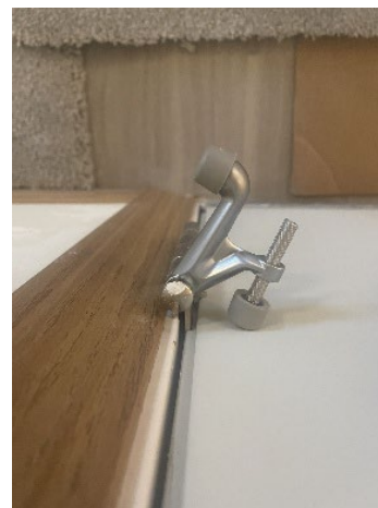
Incorrect Bumper Orientation.
