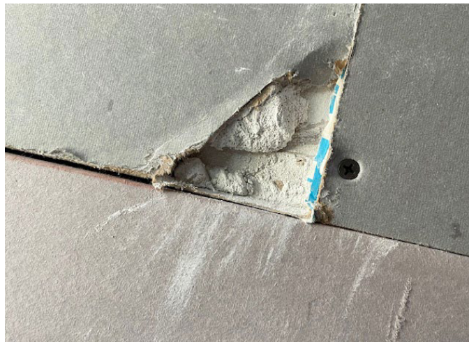
Figure 14-5. Sheetrock Broken Corner.
