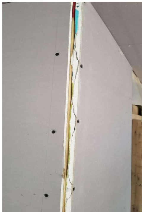
Figure 14-8. Cracking Resulting From One Proud Corner Stud.
