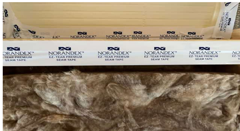
Figure 12-6. Air Gap Between Insulation and Upper Plate.
