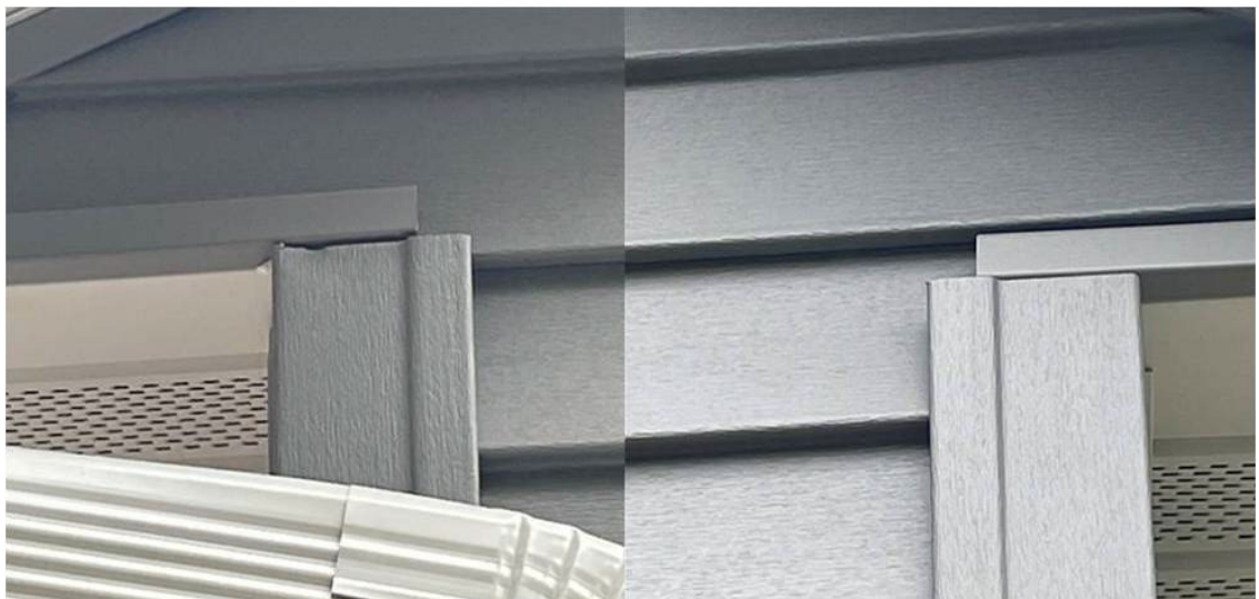
Figure 11-9. Unacceptable J-channel Installation.
