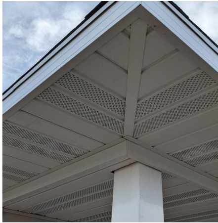
Figure 11-24. Porch Soffit Corner.
