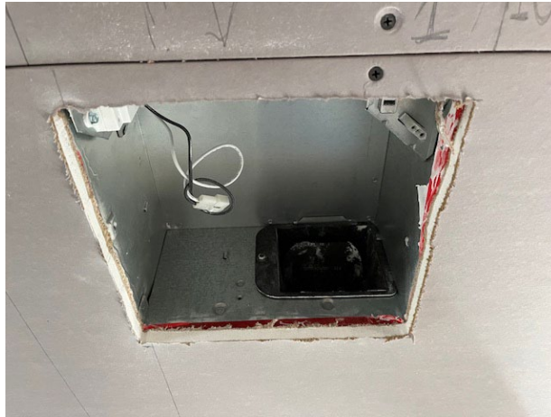
Figure 13-5. Damaged Tape Seal from Spiral Saw Cut-Out for Bath Fan.
