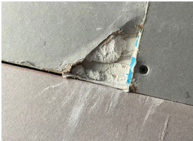
Figure 14-5. Sheetrock Broken Corner.
