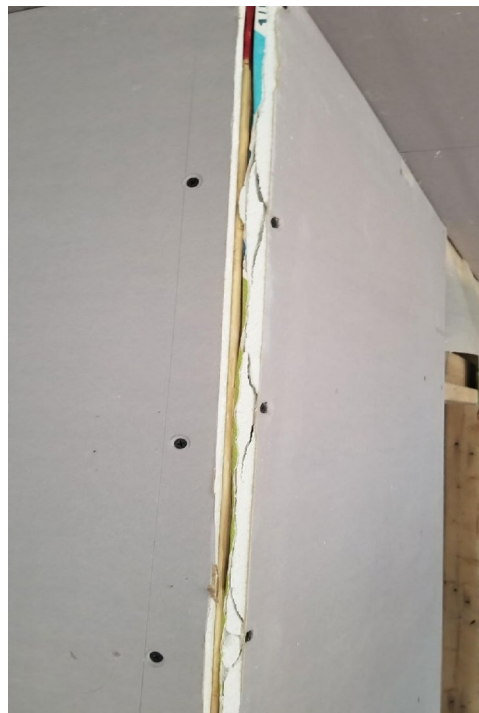
Figure 14-8. Cracking Resulting From One Proud Corner Stud.
