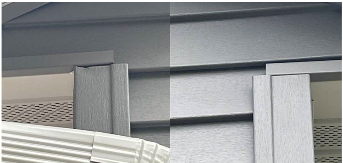
Figure 11-9. Unacceptable J-channel Installation.
