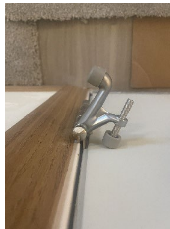
Incorrect Bumper Orientation.
