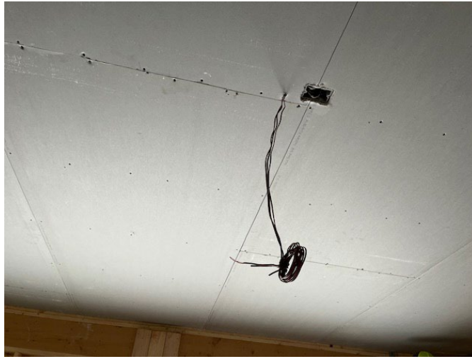
Figure 13-6. Exposing Garage Door Opener Wire.
