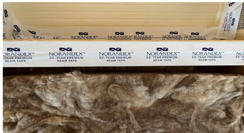
Figure 12-6. Air Gap Between Insulation and Upper Plate.
