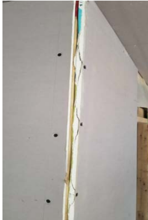
Figure 14-5. Cracking Resulting From One Proud Corner Stud.
