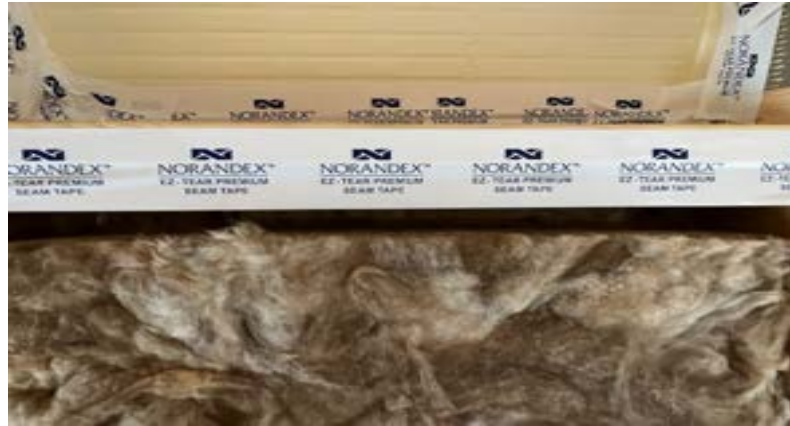
Figure 12-6. Air Gap Between Insulation and Upper Plate.
