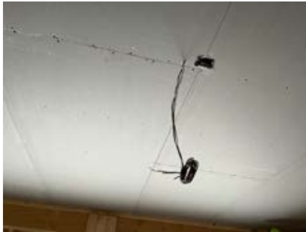
Figure 13-5. Exposing Garage Door Opener Wire.
