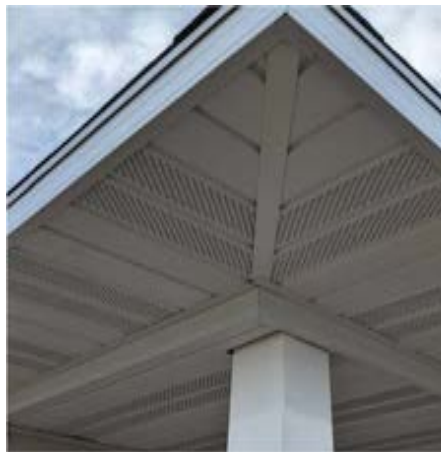
Figure 11-24. Porch Soffit Corner.
