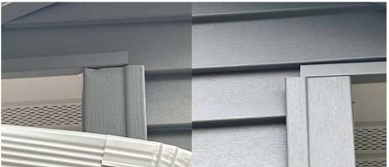
Figure 11-9. Unacceptable J-channel Installation.
