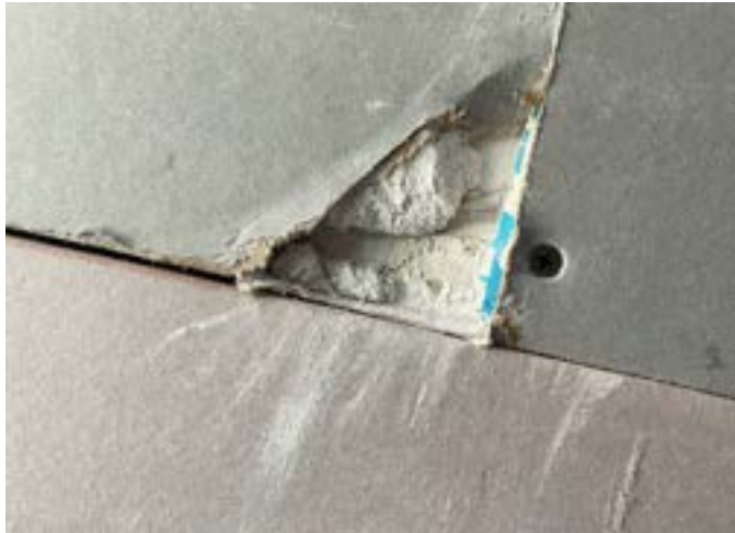
Figure 14-2. Sheetrock Broken Corner.
