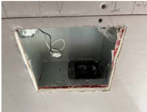
Figure 13-4. Damaged Tape Seal from Spiral Saw Cut-Out for Bath Fan.
