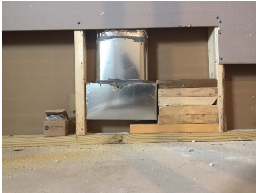
Figure 10-8. Cold Air Return Blocking.
