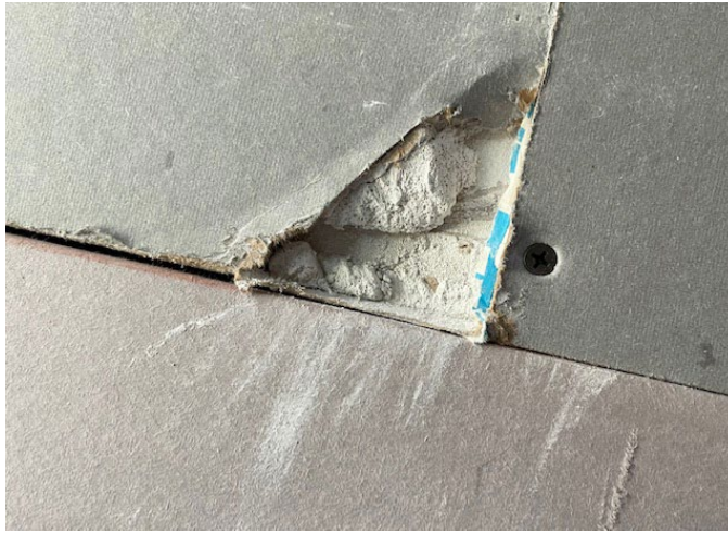
Figure 14-2. Sheetrock Broken Corner.
